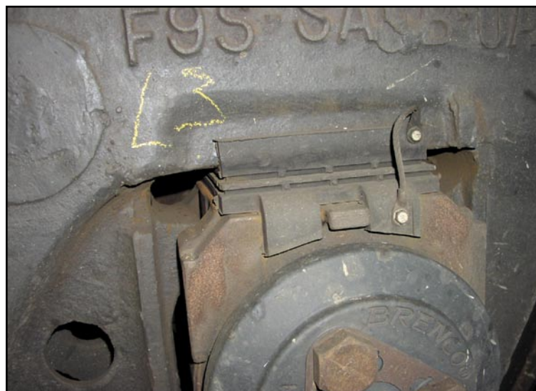
LC Pads are in “like new” condition
